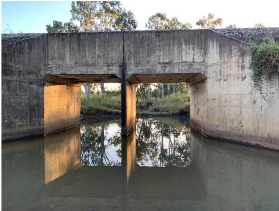
Figure 4.5 - Photograph of the existing railway culvert crossing of Drainage Line 1 at the eastern (downstream) Project boundary
