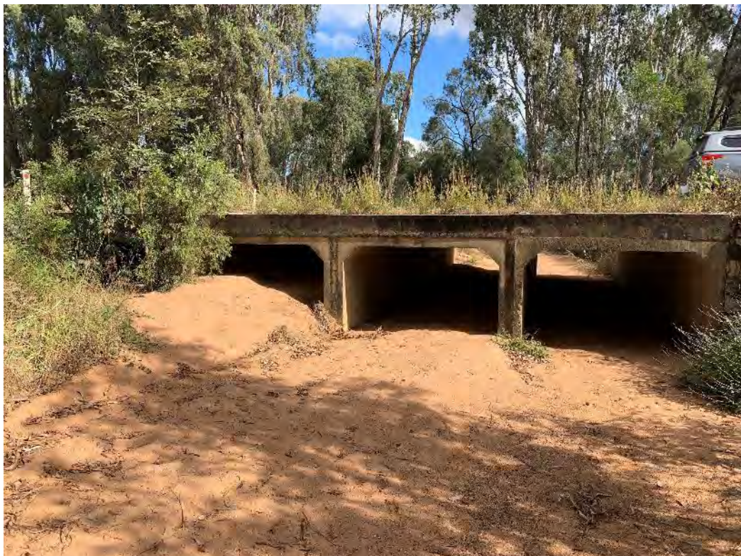
Figure 4.9 - Photograph of Drainage line 7 passing through box culverts under Saraji Road
