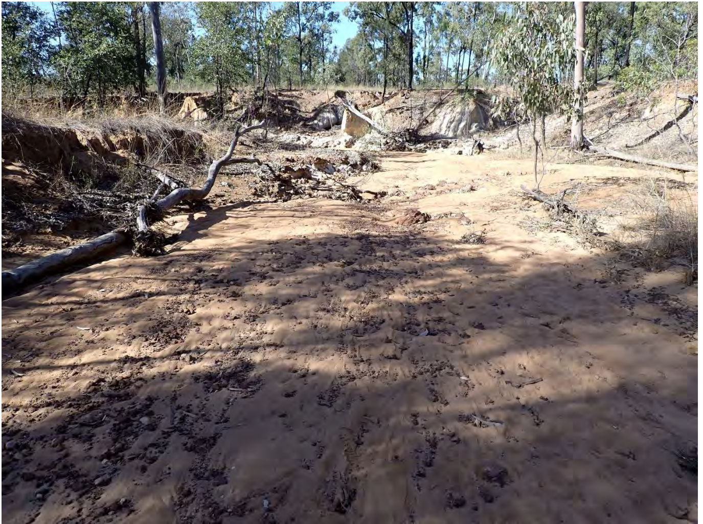
Figure 6-37 Alluvial inspection across Project area. This image shows silty creek bed sediments with presence of weathered profile in the background creek bank and creek bed.
