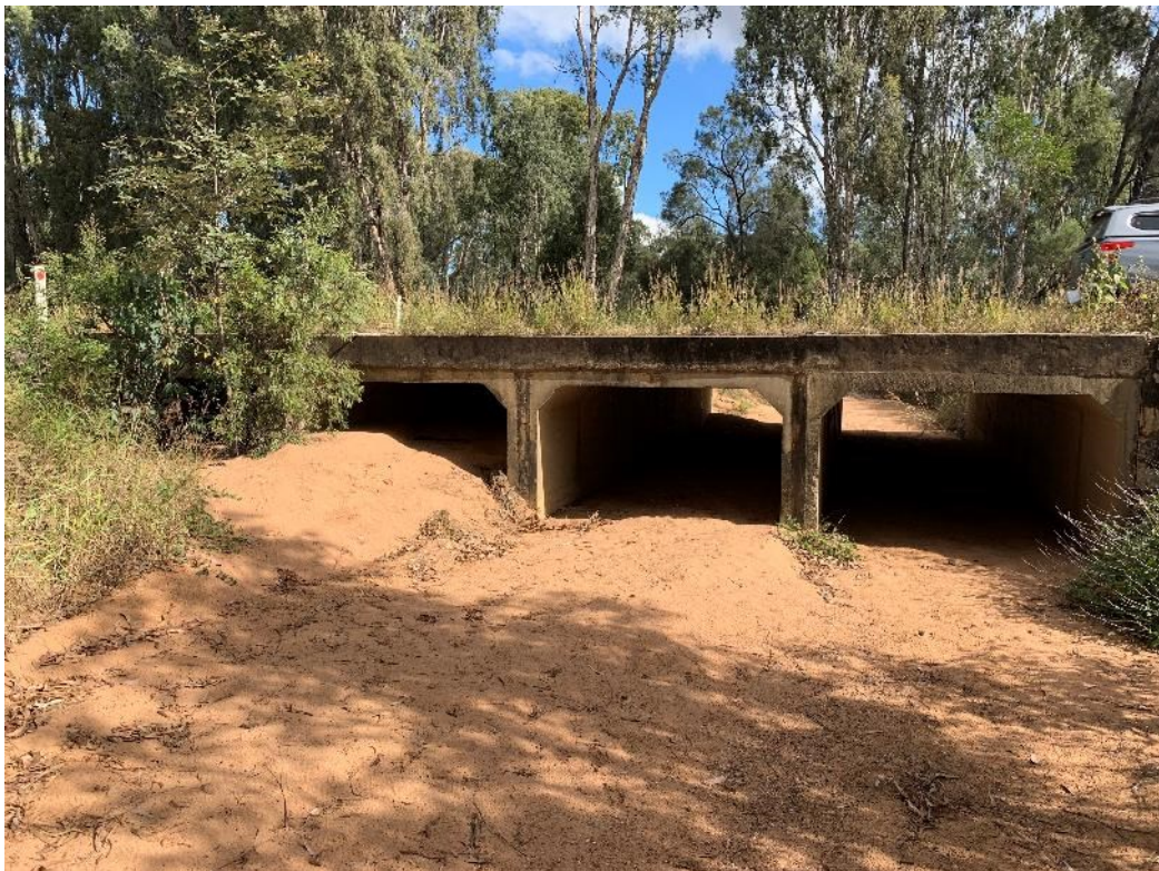
Figure 2.9 Photograph of Drainage line 7 passing through box culverts under Saraji Road
